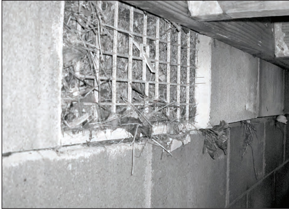
Figure 15. Typical air vent clogged by flood debris
